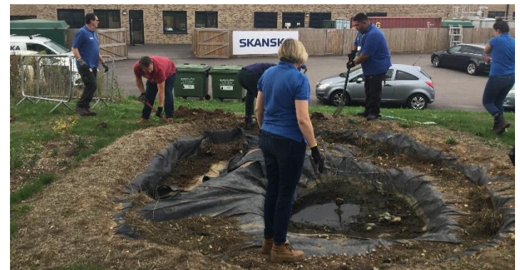
Old pond with torn liner prior to restoration works
